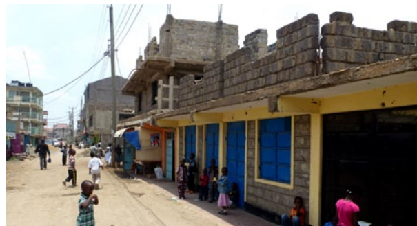
Komarock - suburb in Nairobi. Houses are being built brick by brick depending on the available finances
